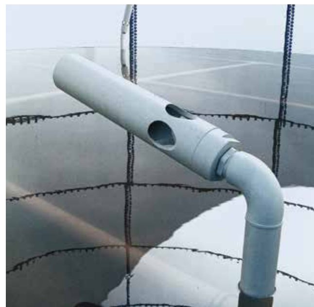
Mixing nozzle in a denitrification
