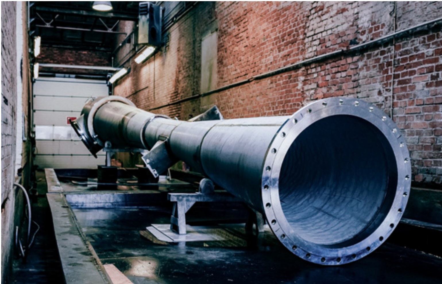
Körting steam jet compressor at the Hanover plant
