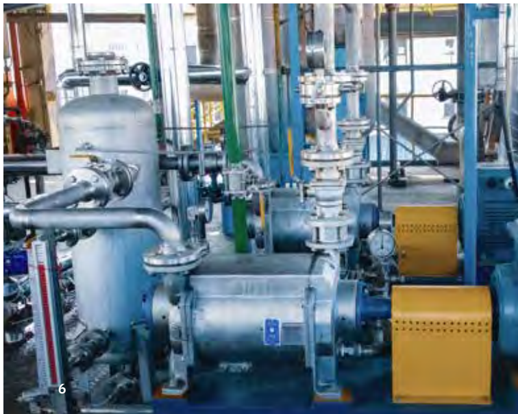
Two water ring pumps connected in parallel as the atmospheric stage for venting
