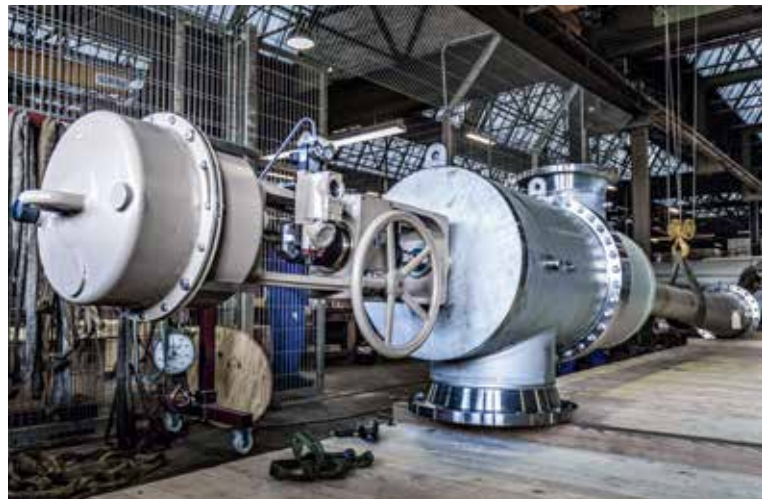
Controllable steam jet compressors with nozzle needle control in the Hanover plant
