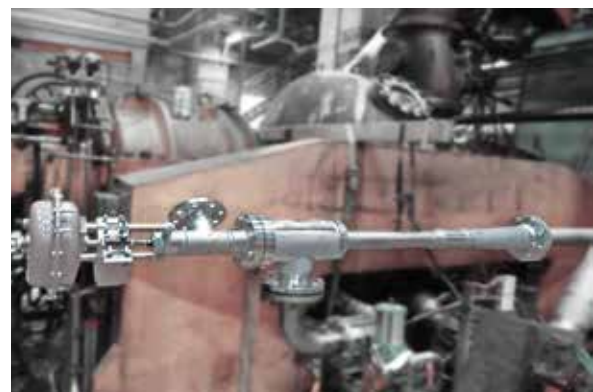
Körting thermocompressor installed on a paper machine
